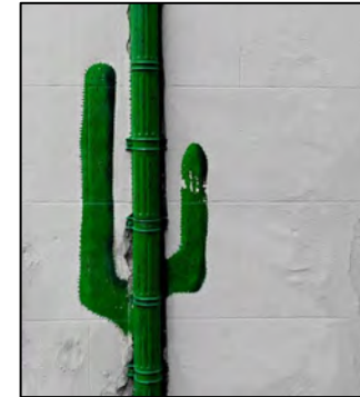
Painted drainage pipe
