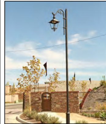
LED lighting with character
